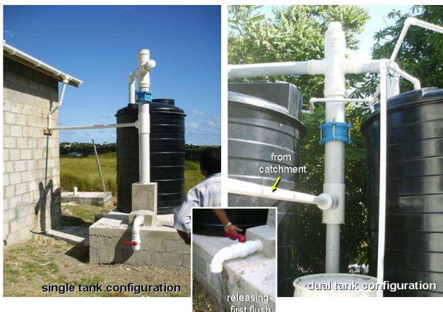
Upflow first-flush filter systems in Antigua
